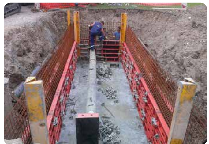
An example of a chamber during construction. Ready-made industrial metal formwork is used for concreting.
