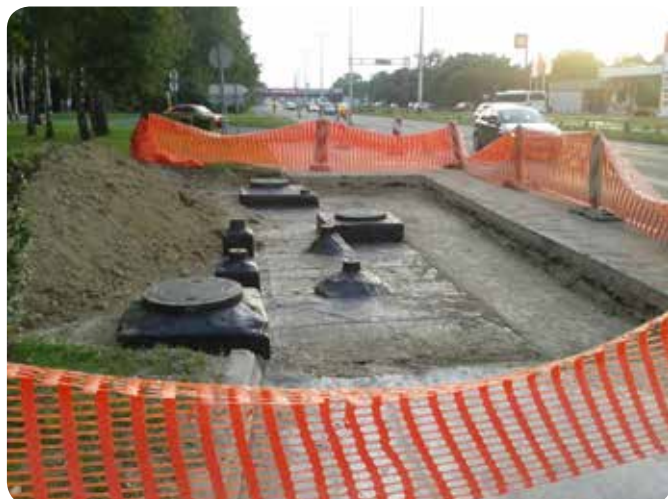
An example of a waterproofing coating of a constructed chamber, just before the final rehabilitation of the public surface on which it was built.
