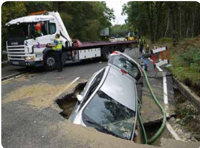
Result of water main burst
