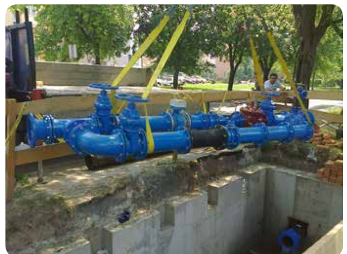
An example of the installation of already combined instrumentation and control equipment inside the inlet chamber with a crane.
