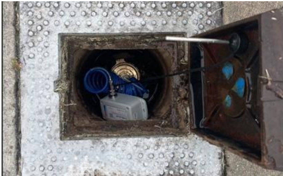
FIGURE B-1 Typical installation of a NB IoT & LTE CAT M1 pressure logger using a modified hydrant cap to access the pipe.
