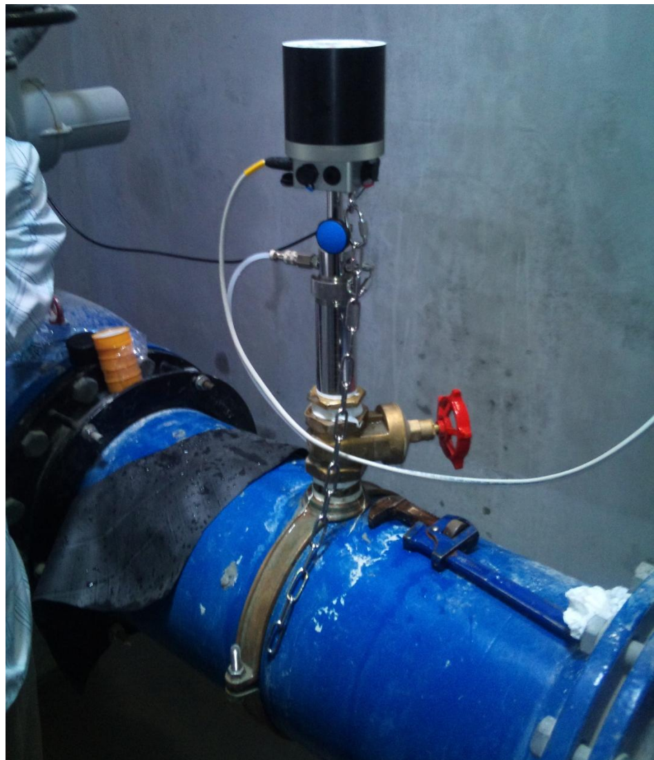
DMA Inlet Chamber in UAE with additional water quality monitoring and Online data communication
