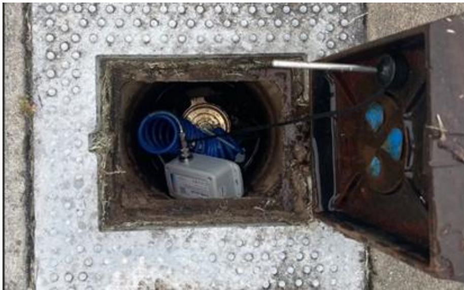
FIGURE B-1 Typical installation of a NB IoT & LTE CAT M1 pressure logger using a modified hydrant cap to access the pipe.
