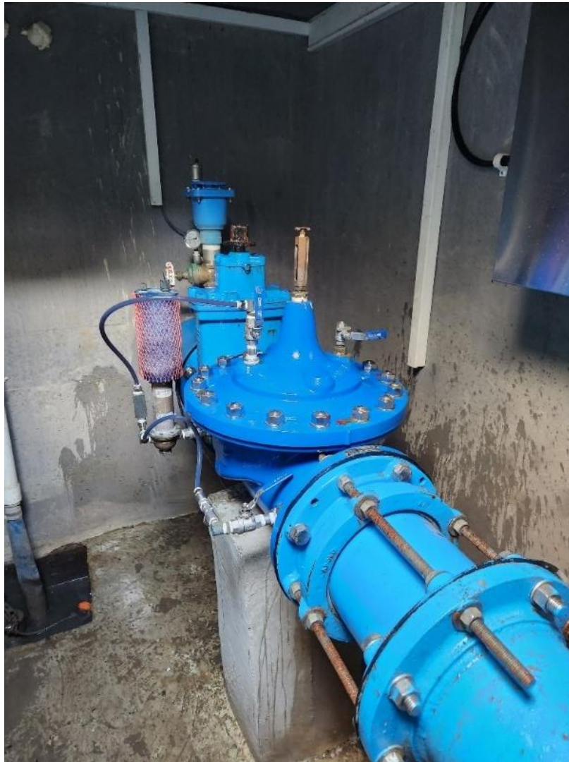
Pressure control and meter chamber, Colombia
