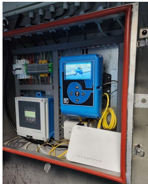
Telemetry and control module of DMA Pressure Control and Meter Station, Colombia
