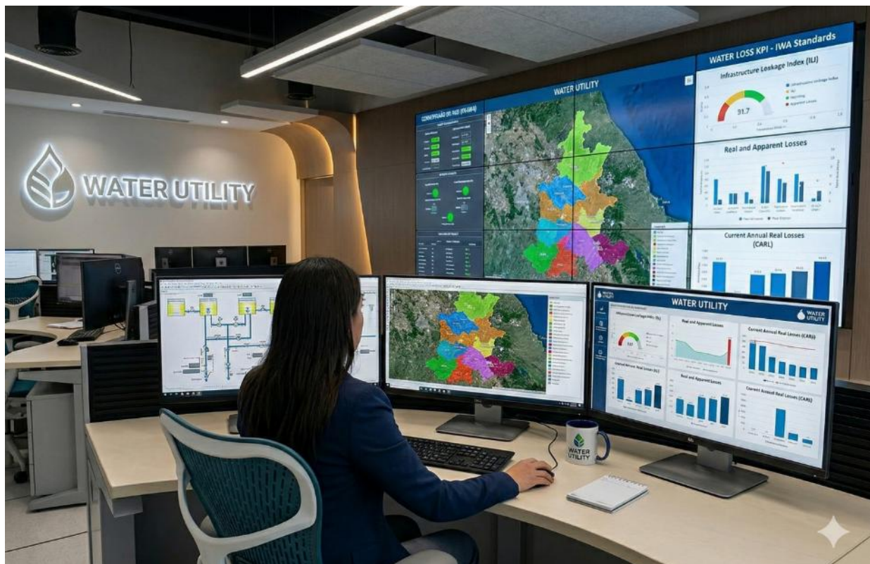
Water Utility Control Center (image generated by AI, Nano Banana, 2026)
